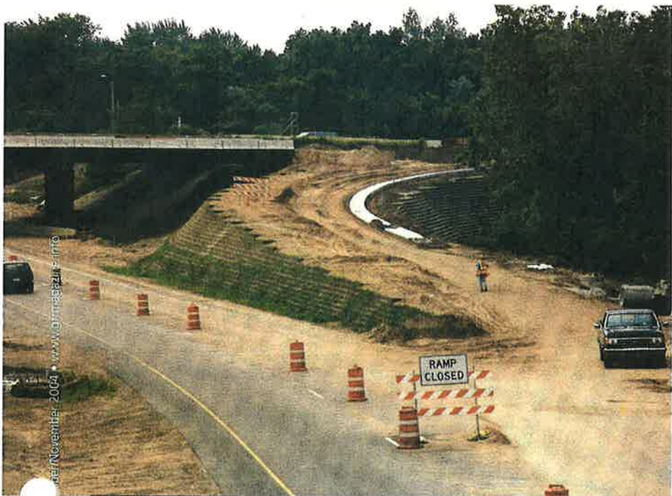
Photo 1. Vegetated geocells on steep slopes. Note how both sides of this highway ramp utilize a "green" approach.
