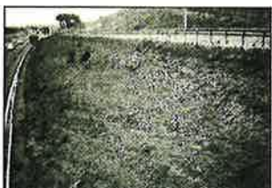
Before: Slope to which hydroseeding was applied. Within two weeks, the cover was completely washed off by heavy rains.
